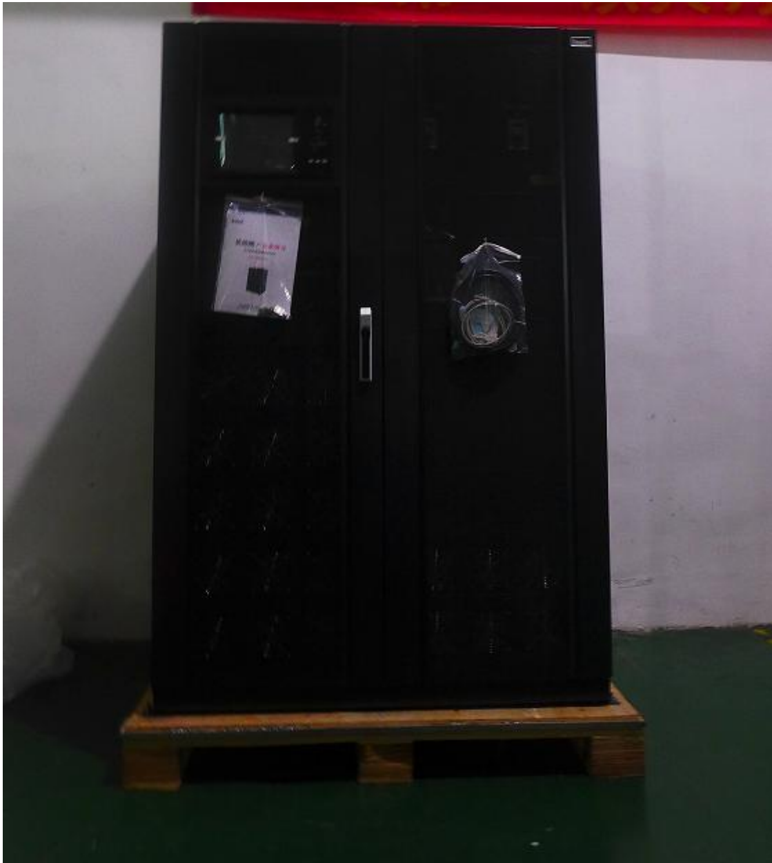
Fig. 1 – Front view for UPS
