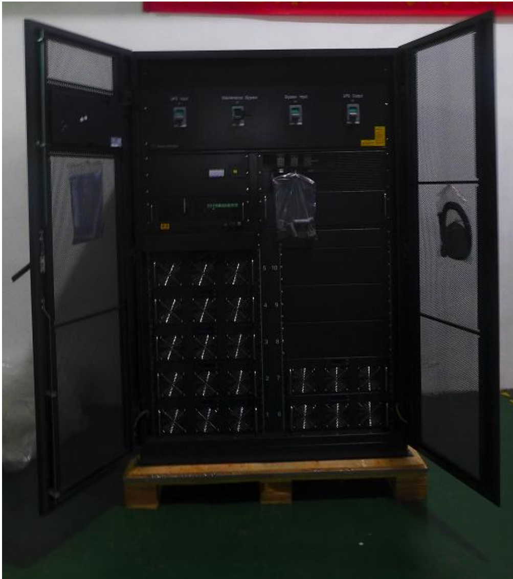
Fig. 3 –Inside view for UPS
