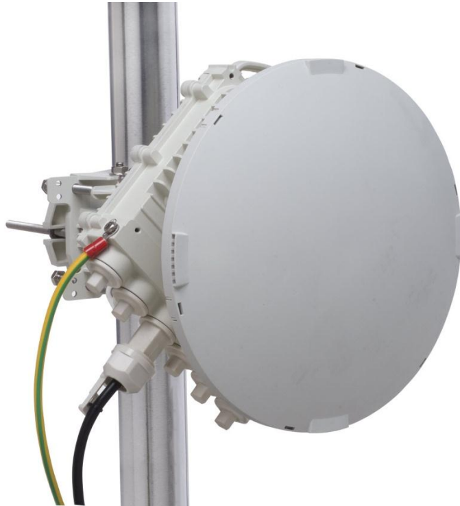
Figure 2-4 ODU with Grounding Cable Connected
