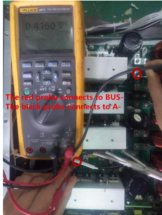
Fig.4-5 rectifier IGBTs detect (b)
